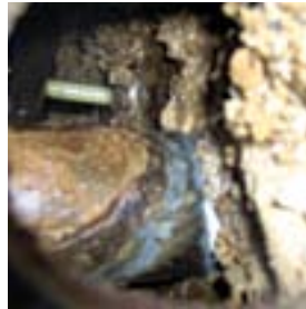
Large deposits of hard scale constrict water flow of this hotel plumbing system.
